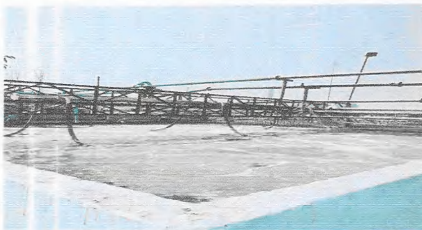
Fig 10 : Aeration Tank I at Meenu Paper Mills Private Ltd
