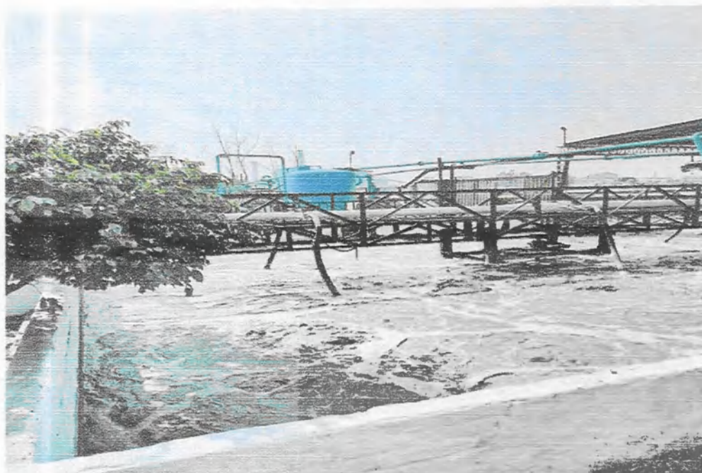
Fig 11 : Aeration Tank II at Meenu Paper Mills Private Ltd
