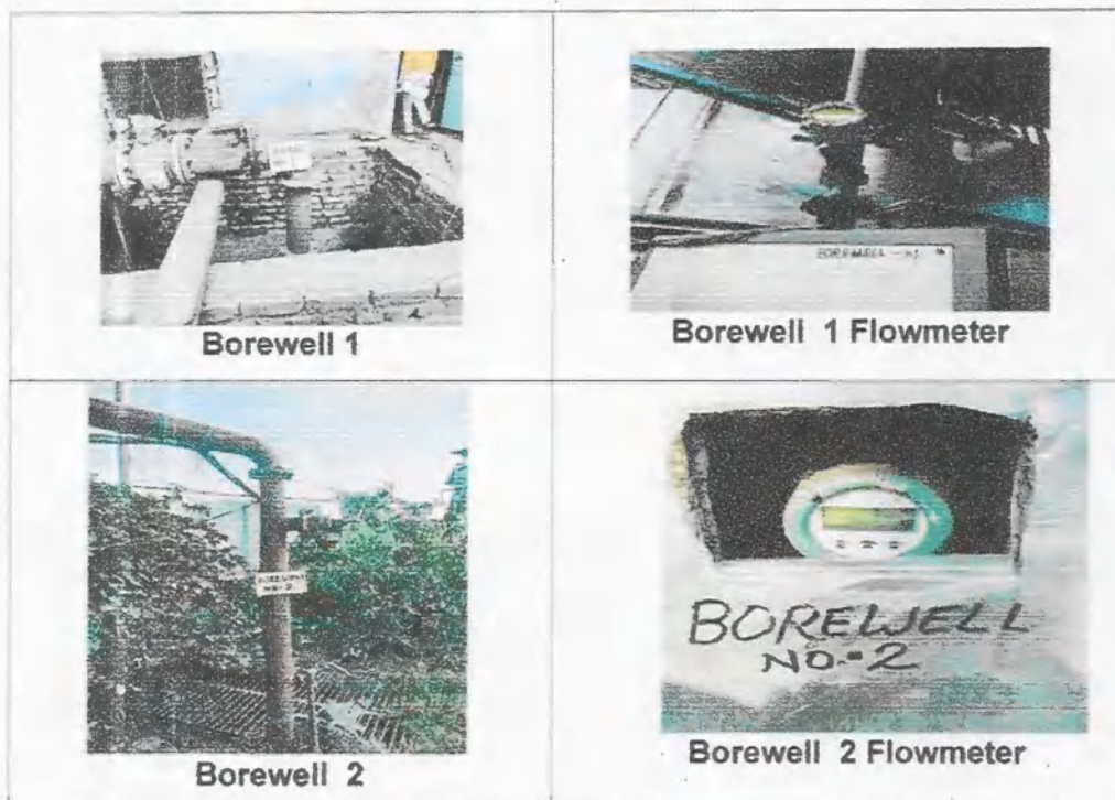
Fig 5 : Borewell & Borewell Flowmeter at Meenu Paper Mills Private Ltd
