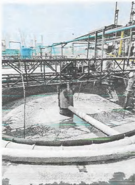
Fig 7 : Equalization Tank at Meenu Paper Mills Private Ltd
